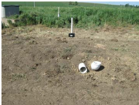
Figure 2. Northwest IA 1 constructed an earthen berm located in front of the VTA outlet.
