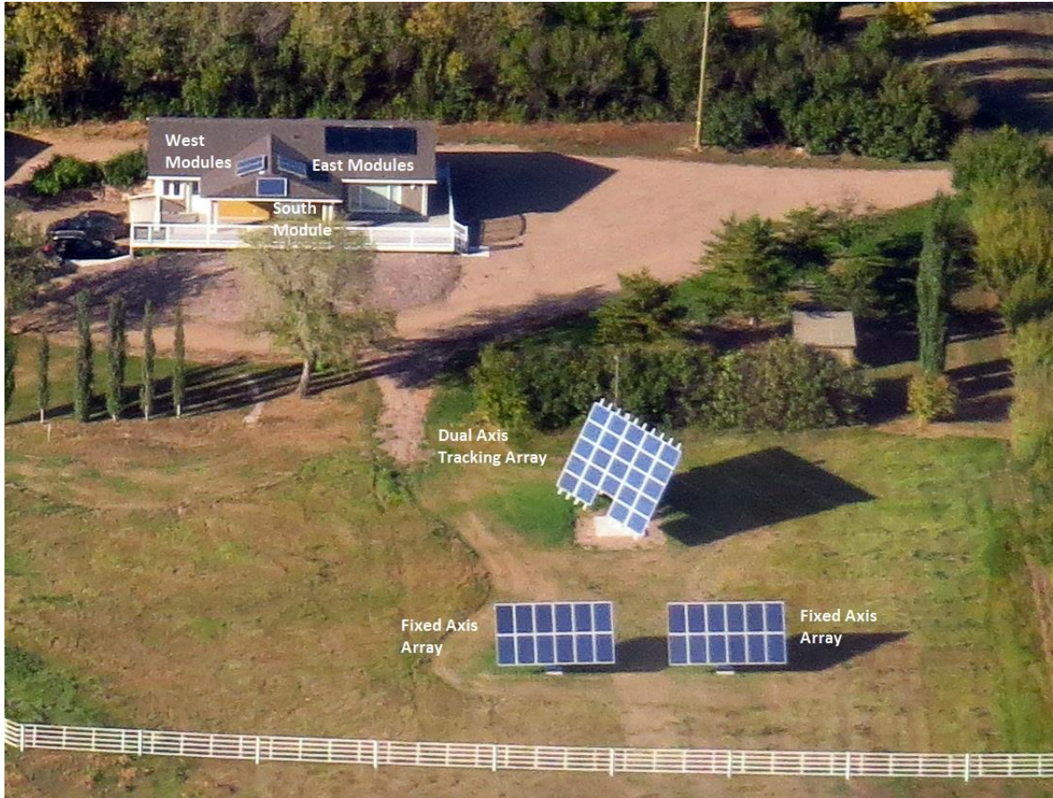
Figure 5: Overhead shot of the RELC facility depicting all of the solar PV systems
